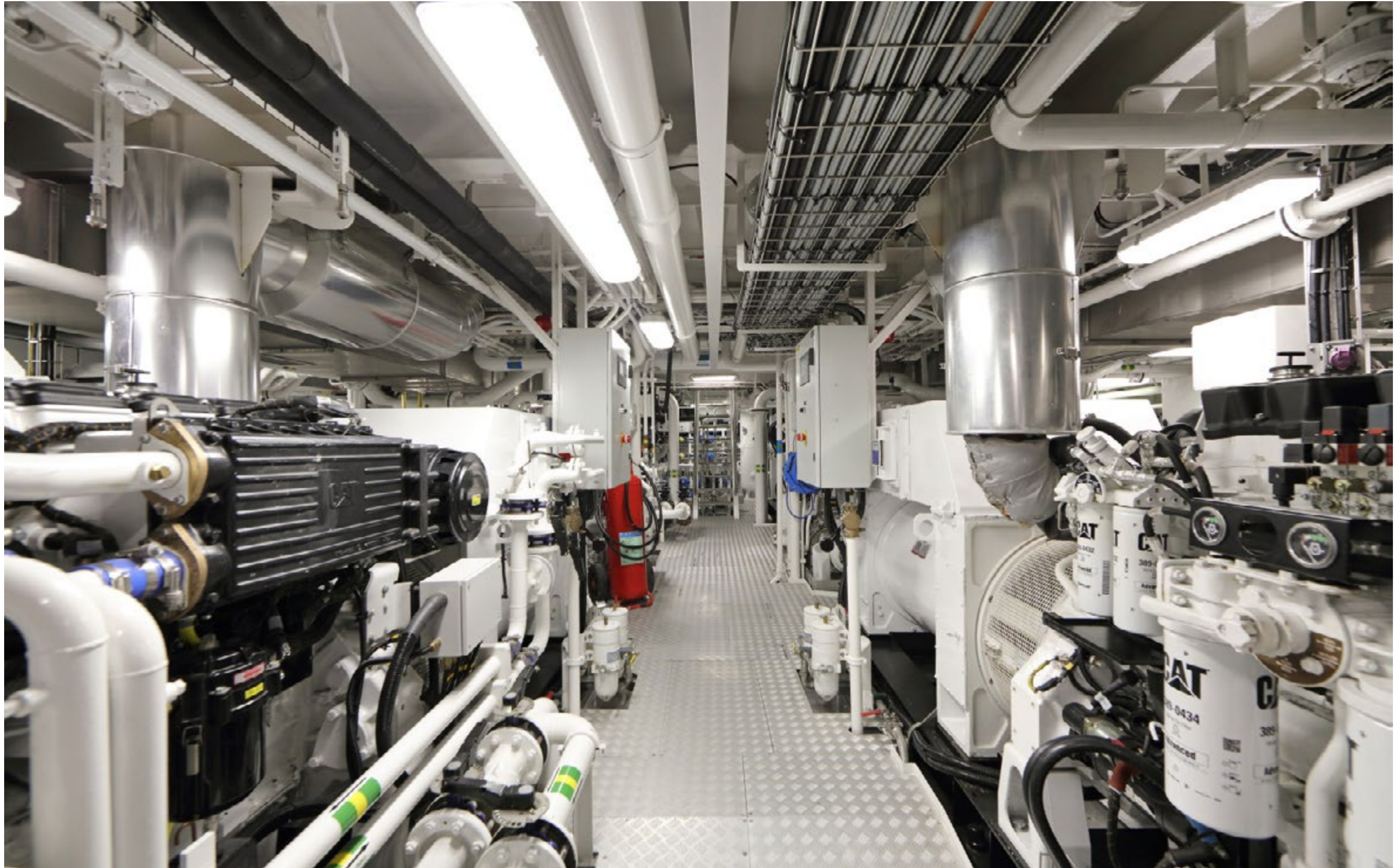
LOWER DECK - ENGINE ROOM
